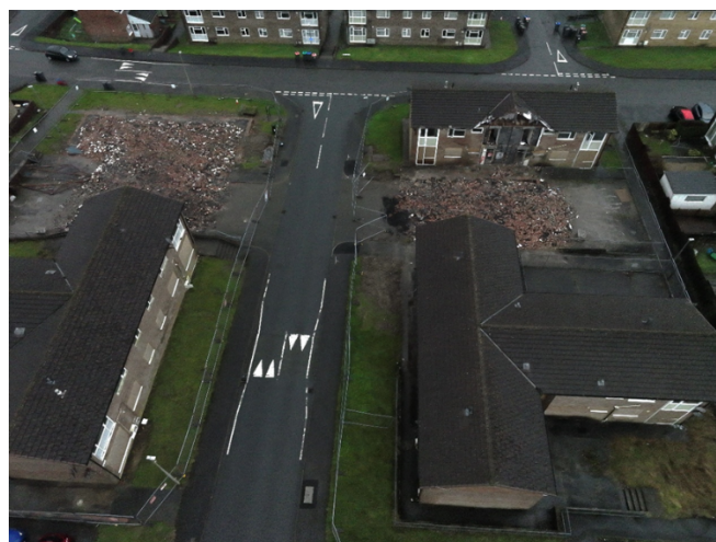
Demolition of out-of-date flats in Ystradgynlais – paving the way for more new Council homes.
